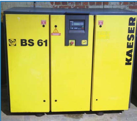
KAESER 50 HP AIR COMPRESSOR
